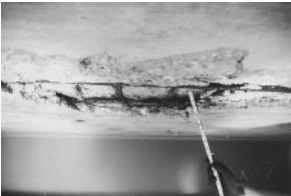
Concrete slab spalling.
